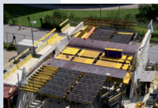
The extensive ceiling areas including haunches were concreted by the building contractor storey-by-storey using formwork tables totalling 450 m 2 with a special sheeting in the required joint grid size
