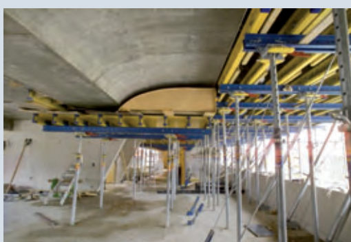
The Ready-to-Use service supplied exact-fit false edge boxes in the desired joint grid size for the interior-running asymmetric haunches.
