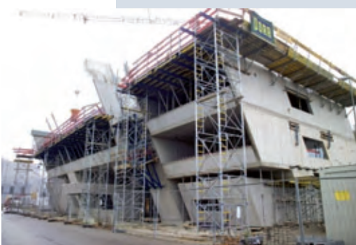
The administration building, which is inclined by 26° to the south, can manage virtually without support frames thanks to the projecting form tables.
